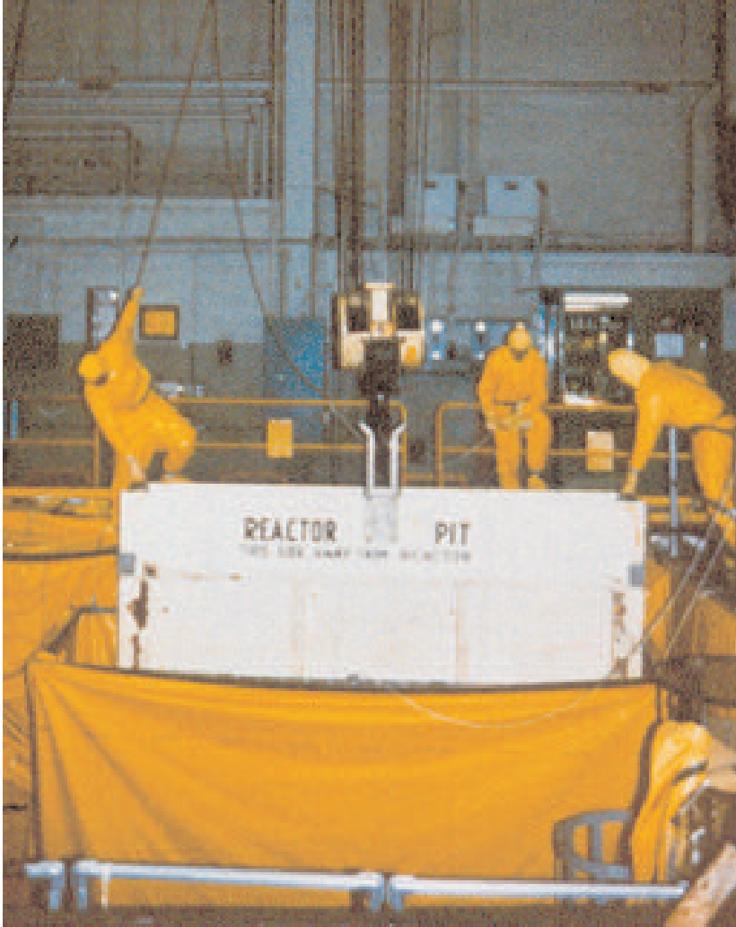
Left: Decommissioning of a pressurised water reactor at Shippingport, USA. It was built in the 1950s and shut down in 1982. Here the wall from the reactor pit is being removed.
