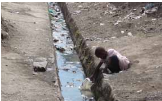
A young girl collects treated water from a cracked supply pipe directly above an open sewer in the slums of Nakuru in Kenya. Since her container is in contact with the contents of the sewer, the water will inevitably be contaminated.
