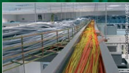
Electrical cables and optical fibres run side-by-side in a data handling centre.
