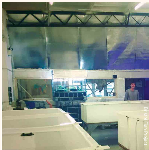
Newly installed tanks at the Bristol Fish Project; eelvers (young eels) ready to grow
