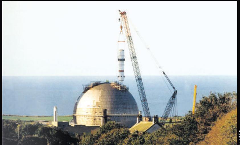
Removing the heat exchanger through the dome of Windscale's advanced gas cooled reactor using the world's largest crane. The metal could not be decontaminated so the entire exchanger has been buried in low-level waste disposal (an engineered trench lined with concrete)
